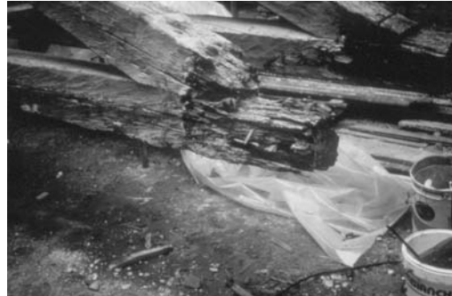
Figure 1 : Localized biological decay (rot) at the end of a roof timber truss, at the connection with masonry walls.
