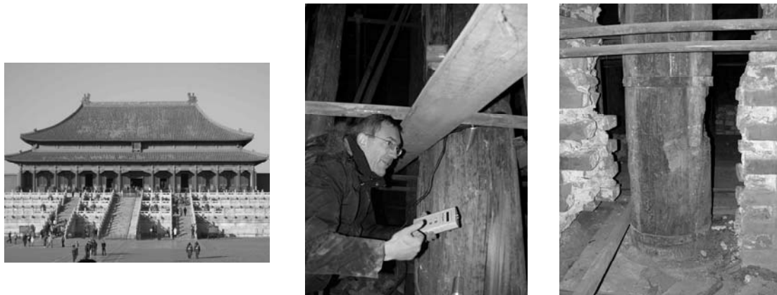
Figure 7 : Expertise of the Forbidden City, Beijing, China. Analyse of the quality of the wooden columns thanks the non-destructive technology Sylvatest-Duo.
