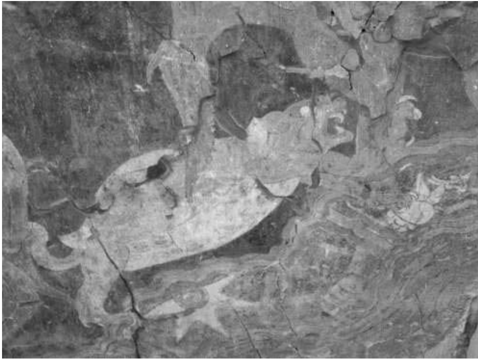
Figure 1 : Typical damage in one of the murals.
