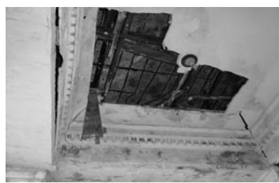
(b) Corroded steel bars in the roof
