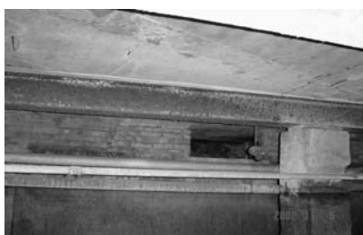
(a) Corroded formed steel sections in the base room
