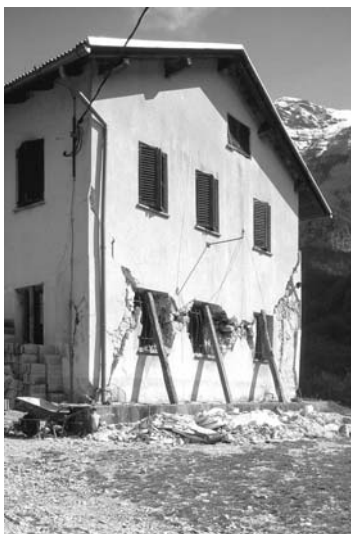
Figure 1 : Typical shear cracks in short window piers
