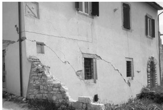
Figure 2 : Shear cracks occur also failure of in long walls
