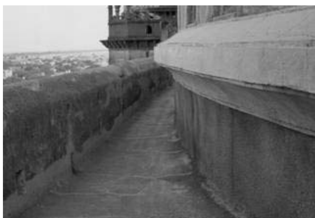
Figure 4 : Hoop cracks in radial direction all around terrace (Base of main dome).
