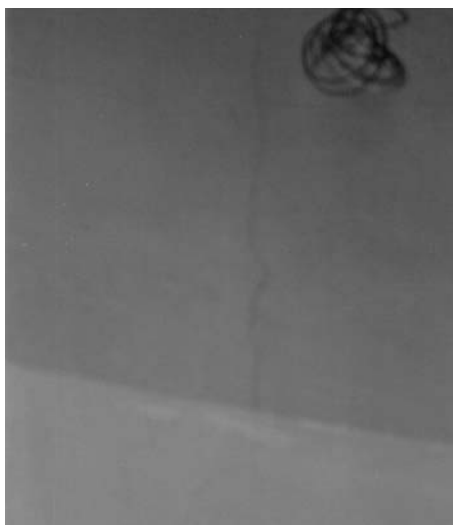
Figure 5 : Showing hoop cracks developed in dome (inner side).
