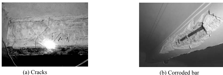
Figure 3 : Craks on a beam and corroded bar in a beam
