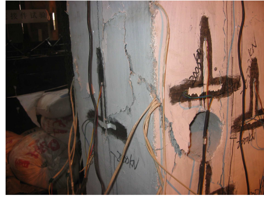
Figure 4: Small-Eccentricity Compression Failure of C4
