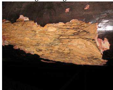
(e) Decayed of wood member in Sichuan Zhaojue Temple
