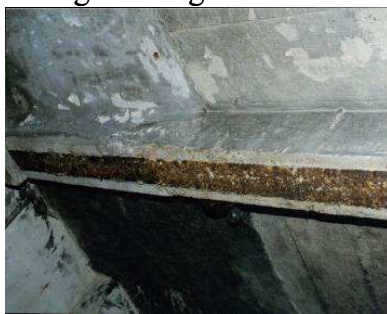
(a) Corrosion of steel in the Building of Bund 18, Shanghai
