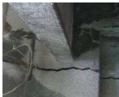
(b) Cracking of structural member in a building in Guangzhou Shamian
