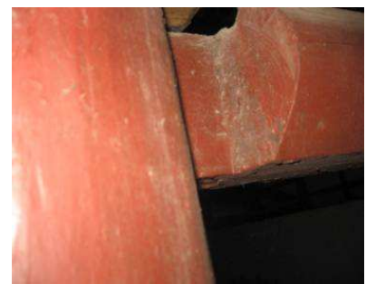
(c) Out of joint in Sichuan Linyun Temple
