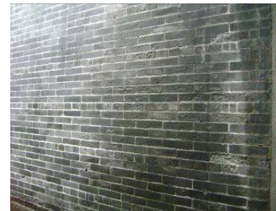
(f) Efflorescence of brick walls in Guangzhou Shoin
