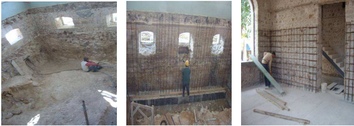
Figure 5: Promoting to cave ground floor of building, Strengthening of ground floor and basement,
