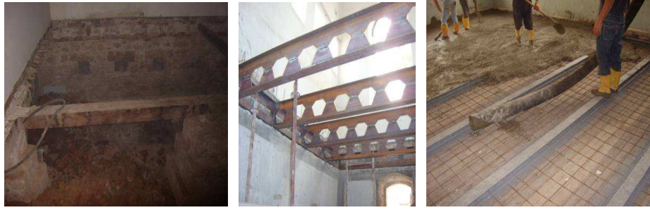
Figure 8: Removing of the damaged floor and making of the new floor with extra steel bars
