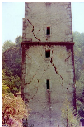
Fig. 7 Bell tower of San Martino – Resiutta (Udine) damaged by Friuli earthquake in 1976
