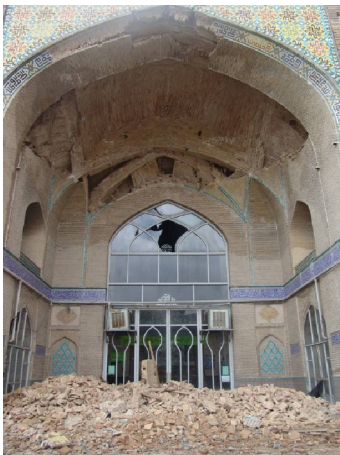
(a) Soltaniyeh Mosque of Brojerd damaged by the Silakhur earthquake (2006)
