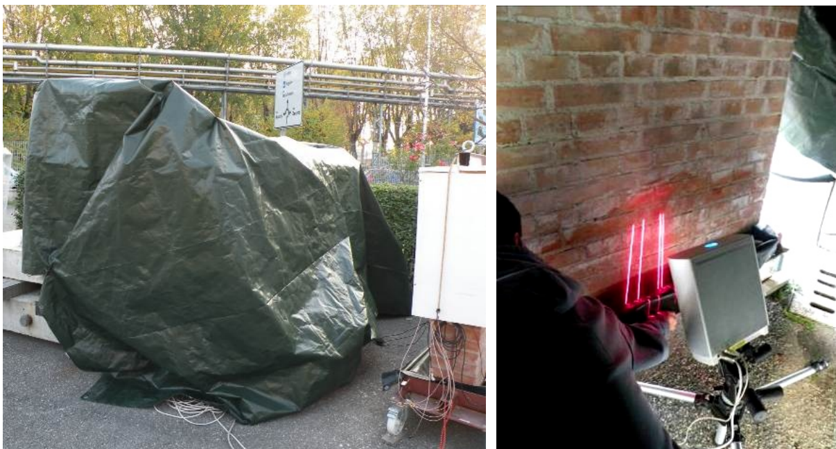
Fig. 4 Masonry wall and surrounding testing area covered with a plastic sheet (left), example of laser scanner survey (right)
