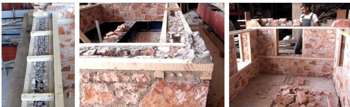
Fig. 7 (a) In-thickness layout of longitudinal and transverse timber elements, (b) Connection of timber elements in the corners of the building, (c) Timber ties and timber frames of openings
