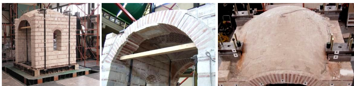
Fig. 5 (a) The strengthened cross vault; (b) Damages in the arch; (c) Damages in the vault [input motion: 450% Irpinia earthquake]
