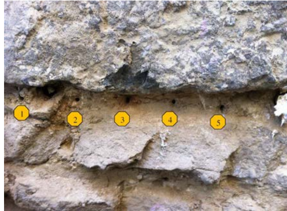
Figure 6: Residential building, Avigliano, panel A, detail after the test.
