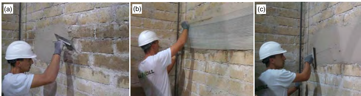
Figure 5. Installation of the mortar-based reinforcement: laying of the first layer of hydraulic lime mortar on the consolidated substrate (a), application of the steel textile (b), and laying of the covering mortar layer (c).
